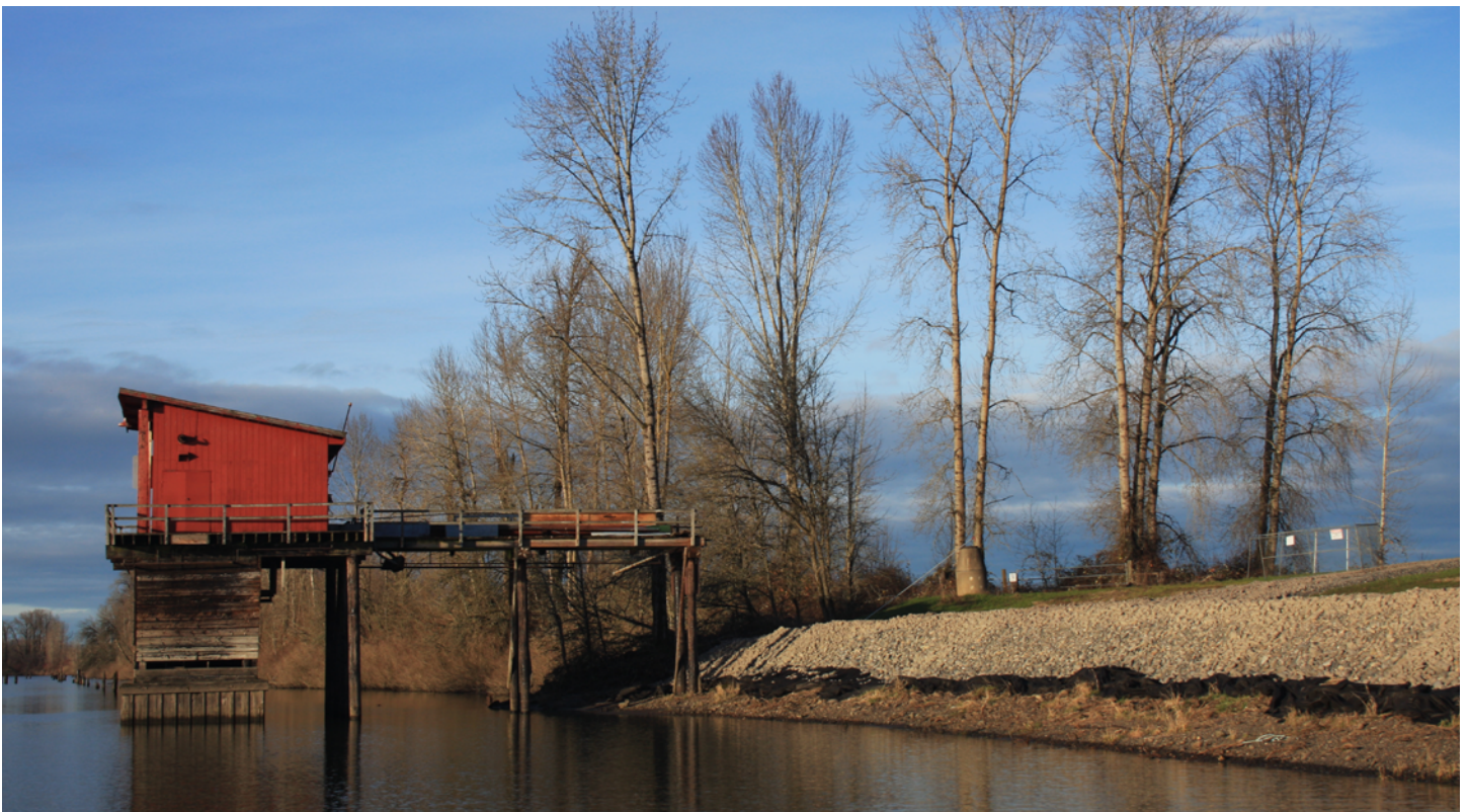
Pumphouse (side view) and river bank.
